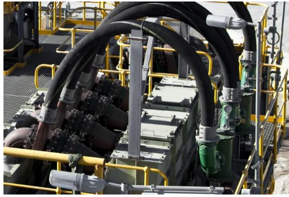
Figure 11. Pumping facility for injecting concentrate
